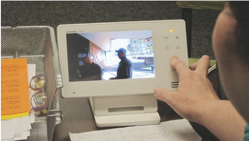
A video intercom from Aiphone was mounted outside Wallace Elementary School's front door. Visitors are instructed to press the intercom's button to talk with the receptionist in the school office. She can see and talk with visitors using a monitor on her desk. If the visitor is approved she remotely unlocks the door.
